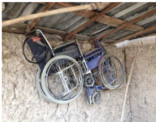
Two unused wheelchairs found hanging from a roof
