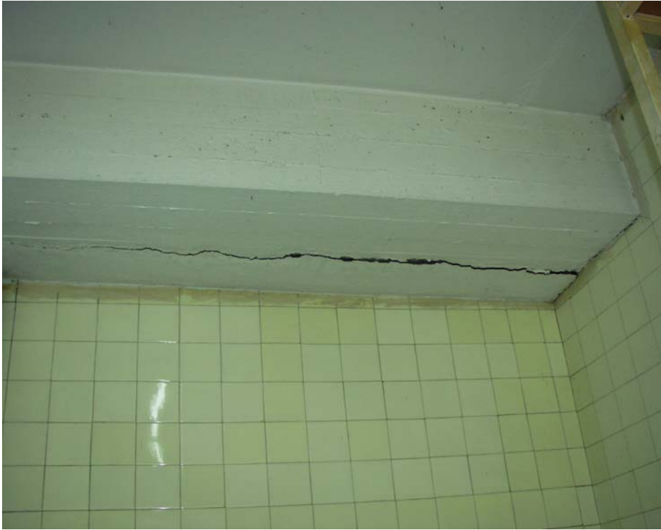
Crack in the beam (basement)
