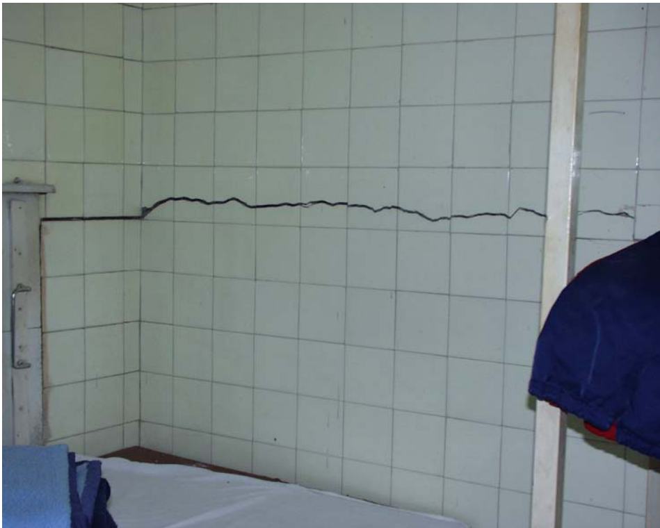
Crack in the basement wall
