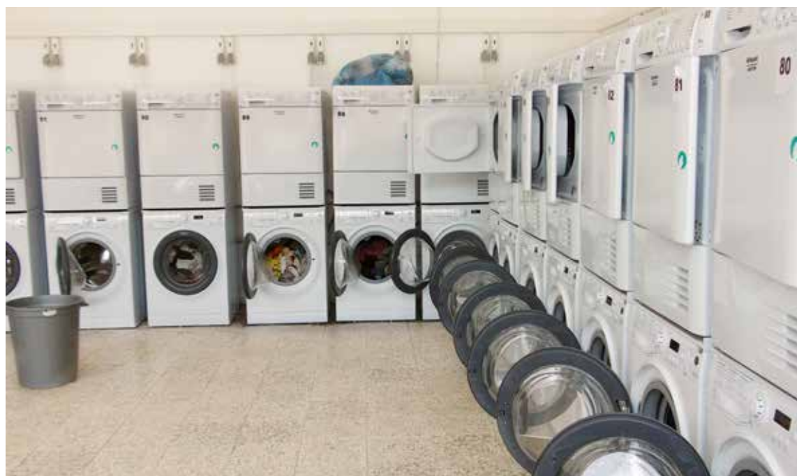
Fig. 6. Laundry facilities at Nizip camp
