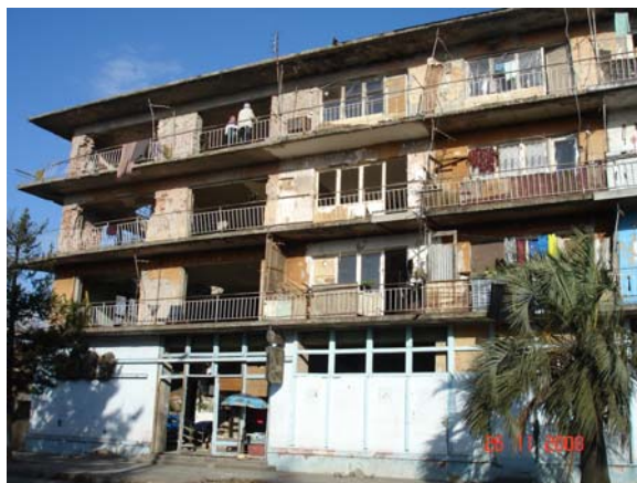
While In Senaki, the WHO team visited a hotel, now functioning as an IDP shelter, which suffered substantial damage during the atrocities in August
