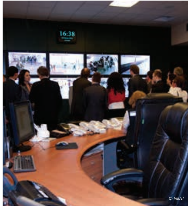
Control center of the Moscow Metro (June 2012)
