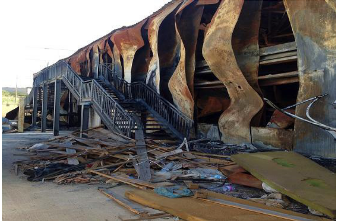
Fig. 9. A pavilion at CSPA after the fire in August 2011
